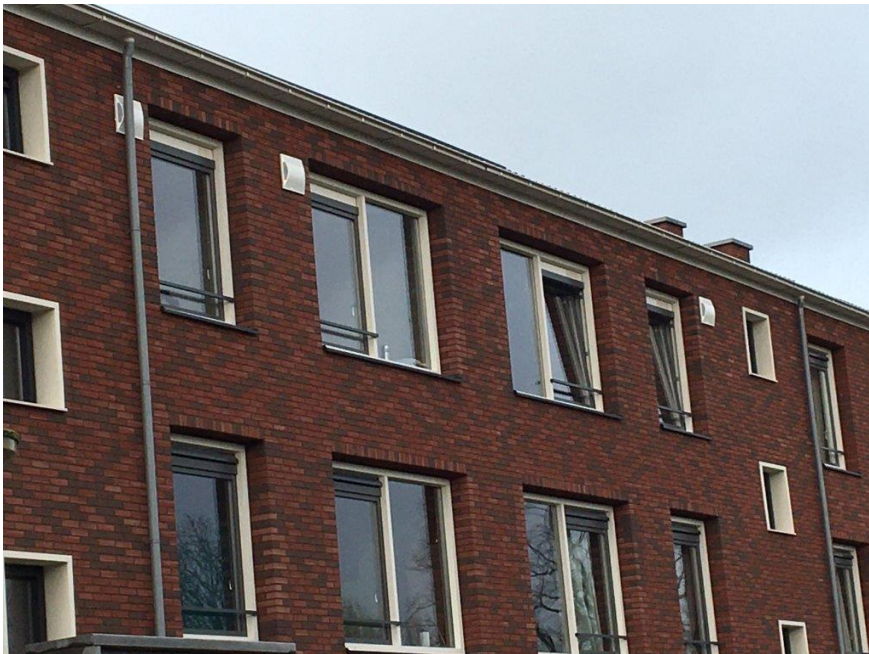
Figure 9: Decentral ventilation units on the external wall of the top-floor dwelling.
