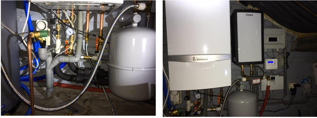
Figure 8: The hybrid heatpump and gas boiler, installed in the attic
