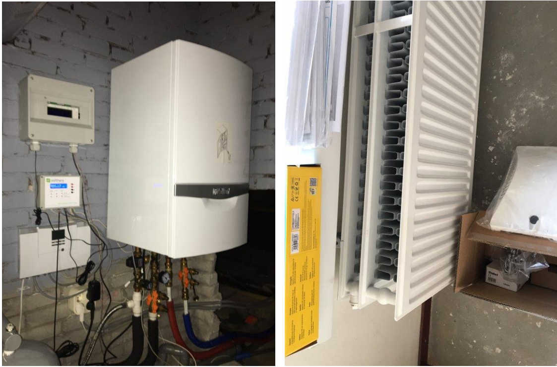
Figure 10: The new heat pump installed in the attic and the new LT radiators.
